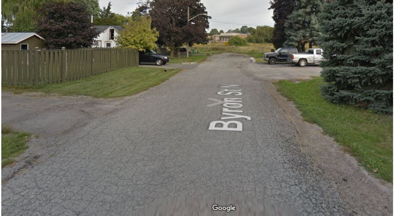
Figure 16 A photo of a road in Very Poor condition
