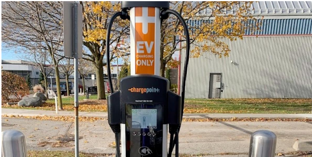
Figure 10. EV Charging Station
