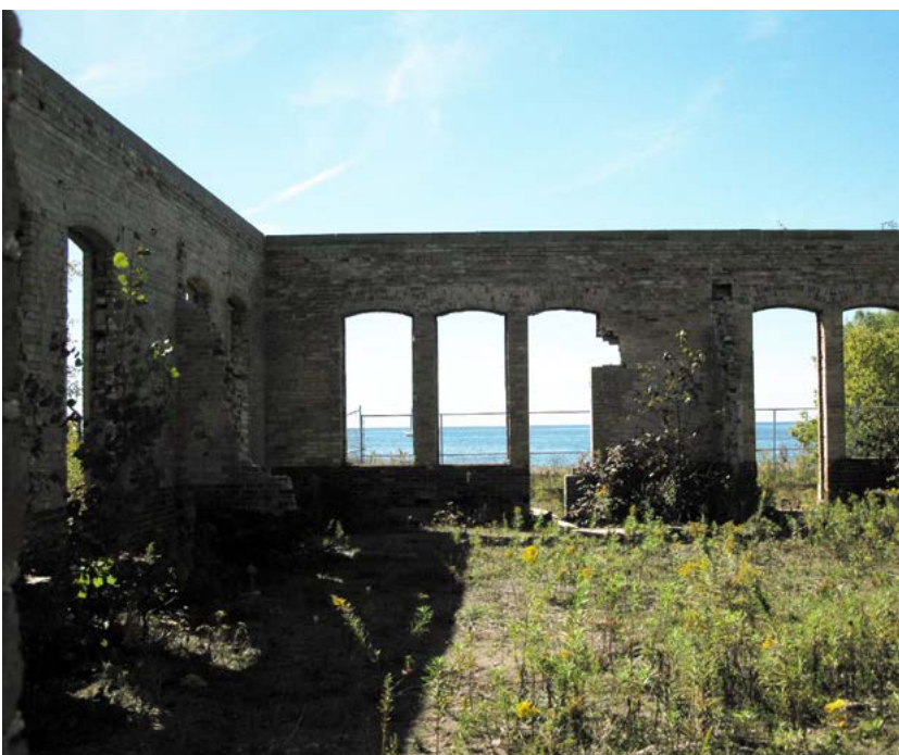
Pumphouse building interior
