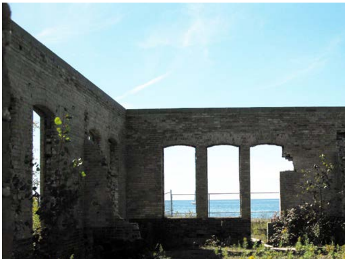
Pumphouse building interior
